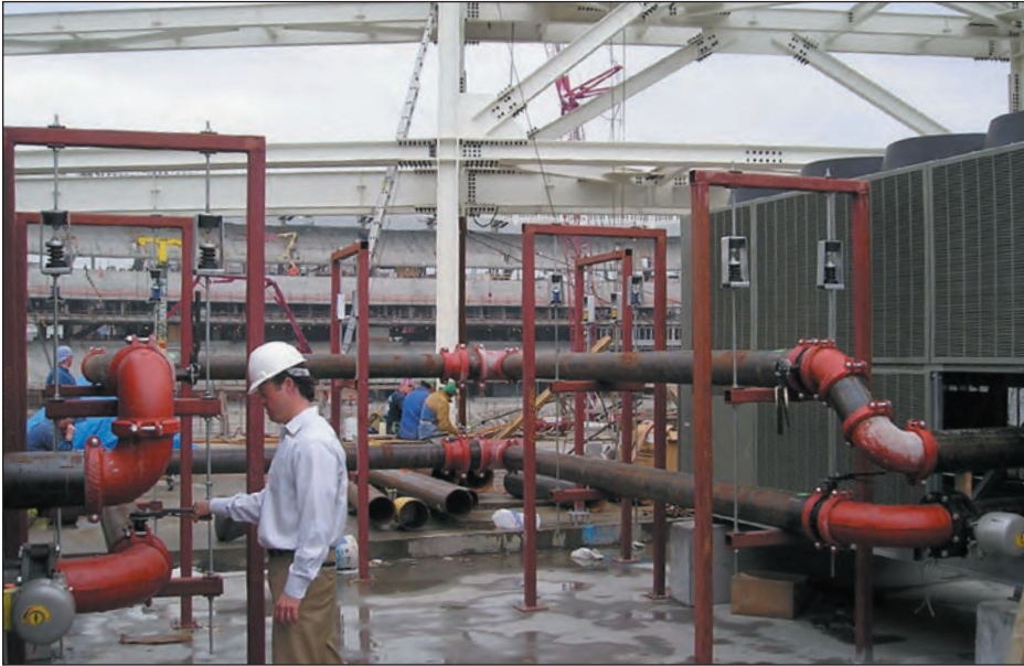
Victaulic Regional Sales Manager Kevin Cahill checks out the Victaulic Style 07 Rigid Coupling, fittings, and elbows and Vic-300 MasterSeal butterfly valves installed by F.W. Sims, Inc. on the air cooled chillers at the new Yankee Stadium.
